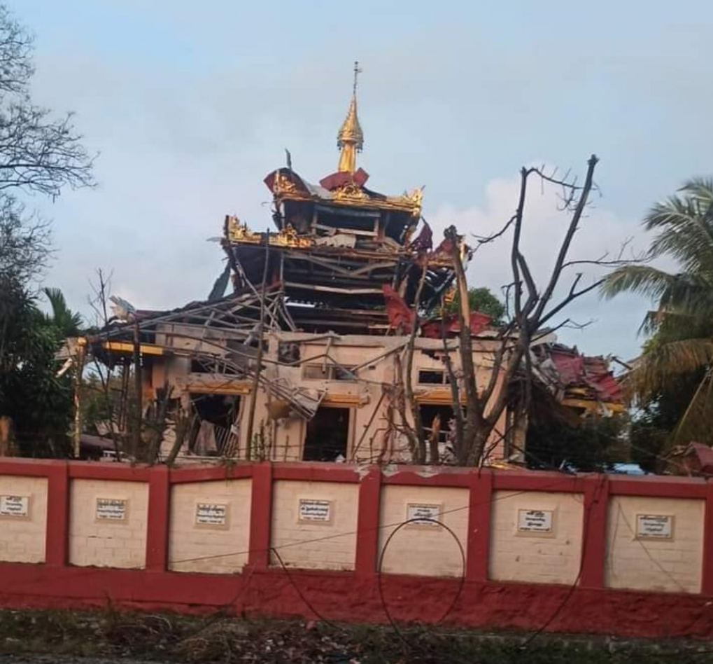
Photo: Additional damage and destruction as a result of fighting in Loikaw, Karenni State.
